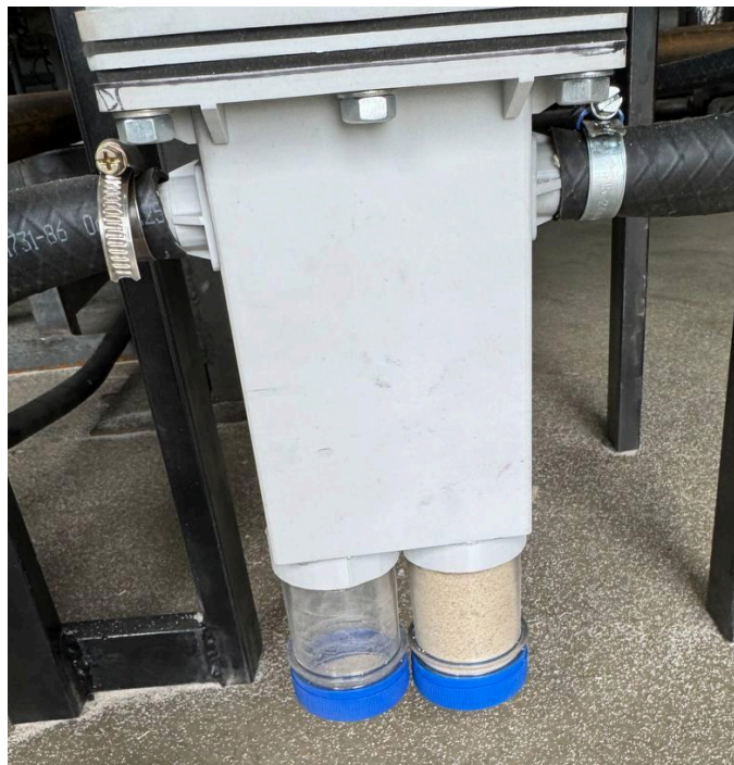
Figure 45. Sand leakage to the air plenum of the lower loop seal.
