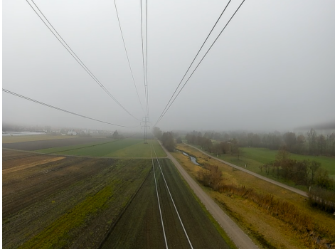
(c) Real UAV photograph: foggy rural corridor with transmission tower and multiple conductors.
