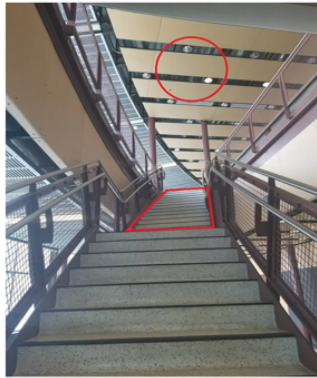
Figure 3.5 Inaccessible light fixture above the stairs
