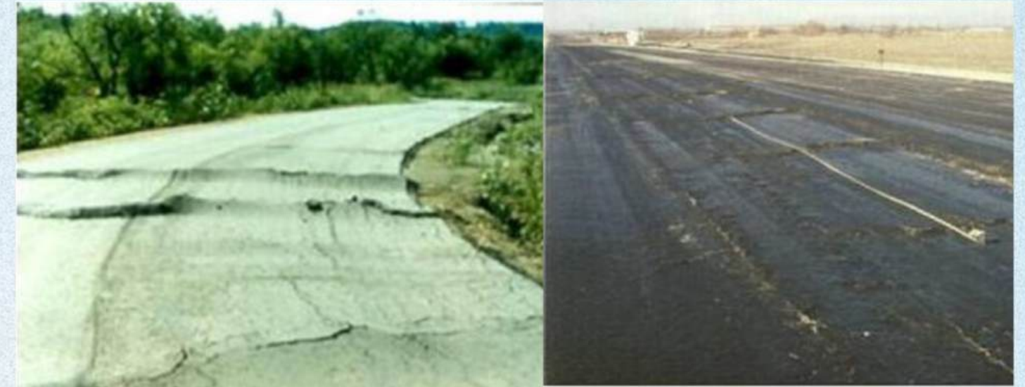
Fig 3. Sulfate induced heaving of a pavement in India [2]
