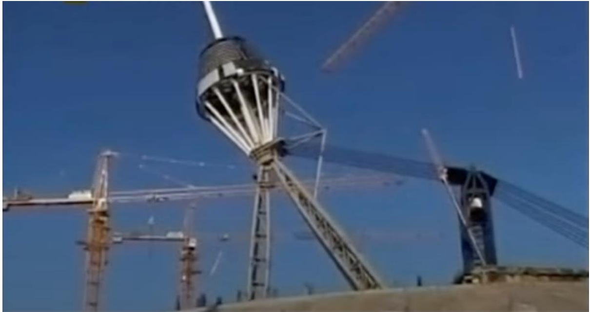
Figure 46: Khan Shatyr construction process of lifting a steel tripod with hydraulic press and mounting it into place. State archive
