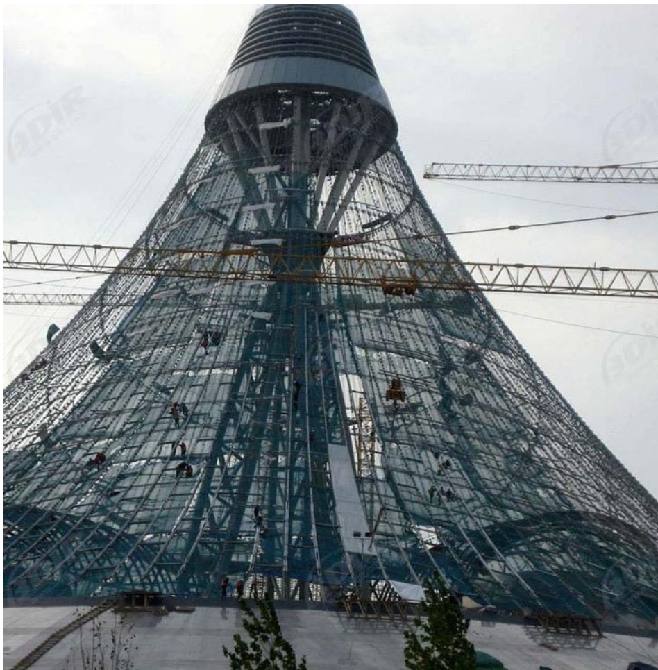
Figure 51: Construction process. Steel cables (spider web) have been mounted on to Khan Shatyr. Construction site documents
