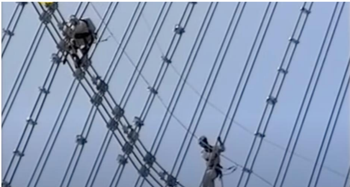
Figure 49: Climbers are mounting steel cables during the construction process. Construction site documents
