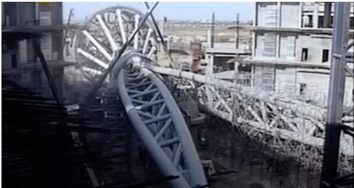
Figure 45: Khan Shatyr construction process of lifting a steel tripod and mounting it into place. Online documentary
