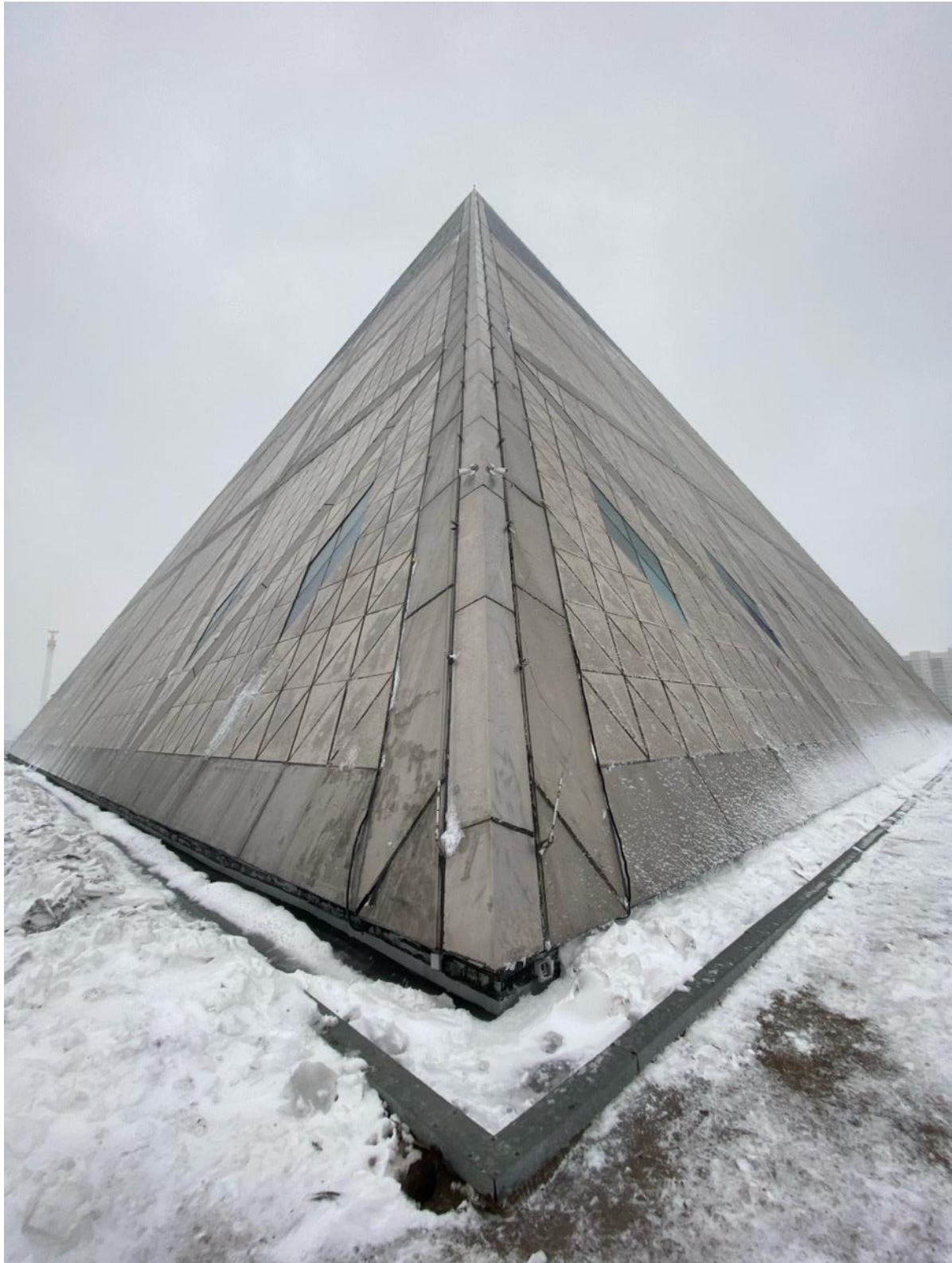
Figure 28: Photo by the author during the winter rain and snow fall drainage system of the Pyramid (2024)
