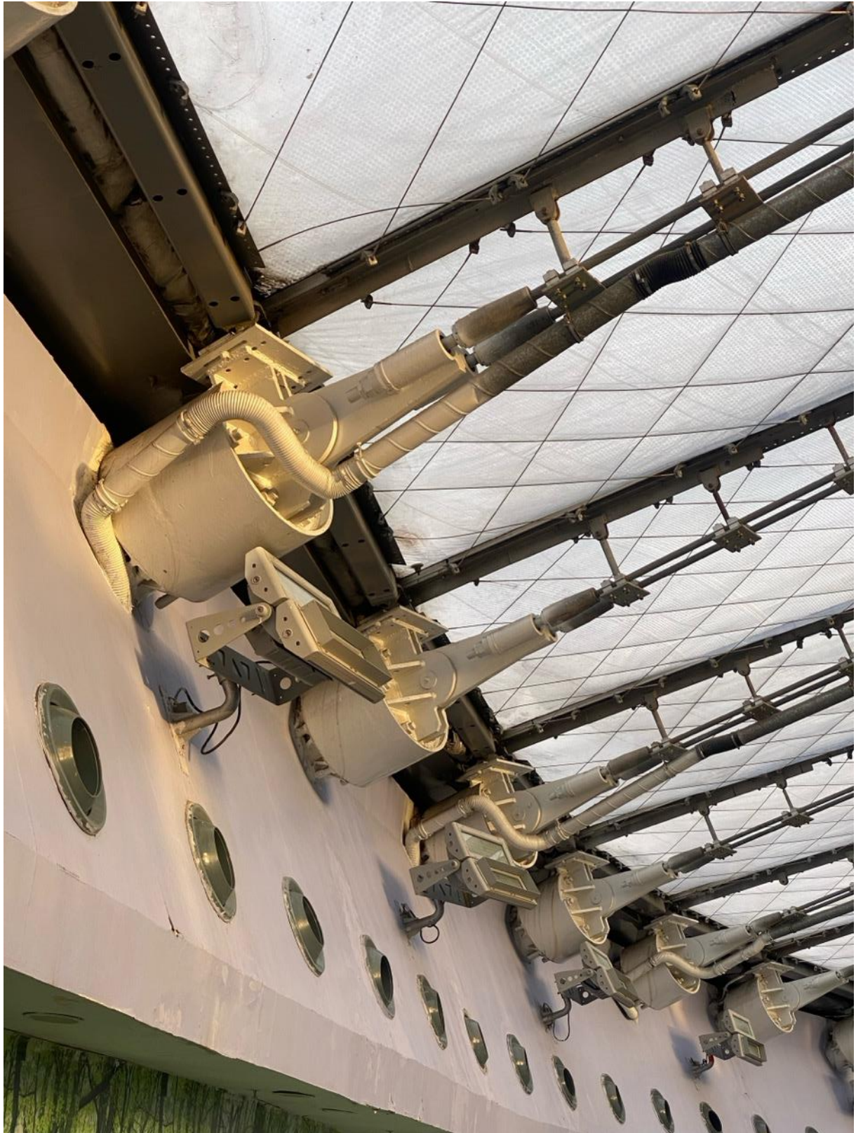
Figure 52: Steel cables attached to the concrete platform. Air vents and air supply to the ETFE layers to keep them filled with air. Photo by the author 2025
