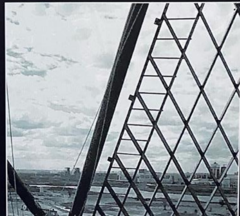
Figure 8: Construction process. Assembling the “Cradle of the world” made of steel structure prefabricated in Britain and assembled on site in Astana. Photo by the author 2025
