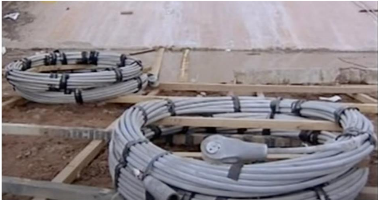
Figure 50: Steel cables for Khan Shatyr that were manufactured in Germany have arrived on to the construction site in Astana. Picture from construction documents
