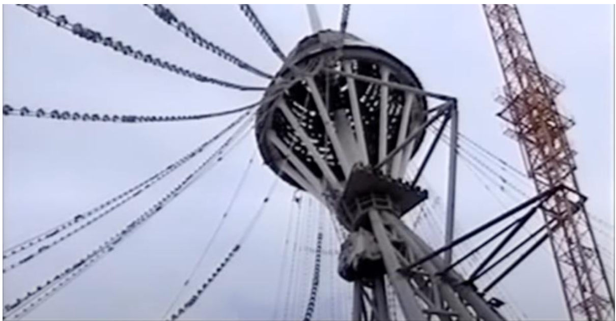
Figure 47: Khan Shatyr construction process of mounting steel cables onto a tripod. Online documentary
