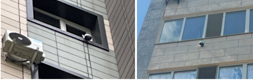
Figure 17. The BlueSky installation in E.B. household (left) and D.K. household (right).
