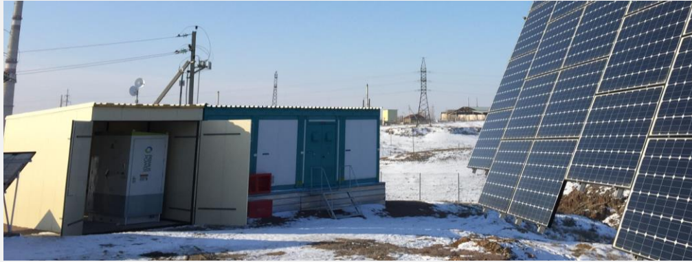
2 MW solar farm in Kapchagay
