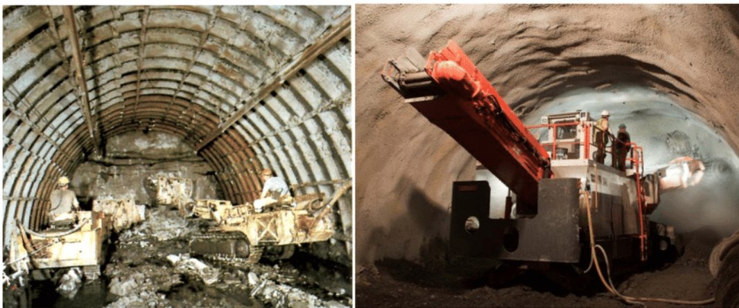
Figure 1: Comparison of Roadheader Machine Excavation with Drilling and Blasting in a Mining Environment (Krzysztof & Piotr, 2019).
