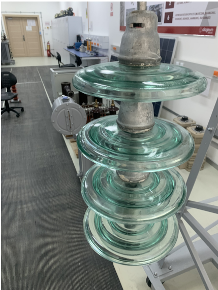
(b) Glass insulator
