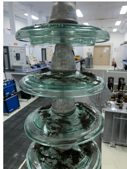
(b) Glass insulator
