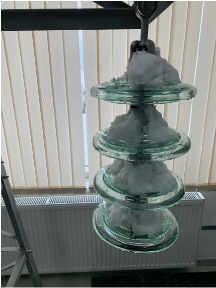
(b) Glass insulator
