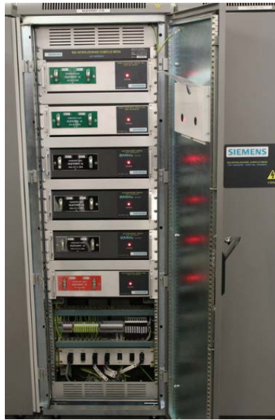
Figure 2.10: Equipment in Solid State Interlocking
