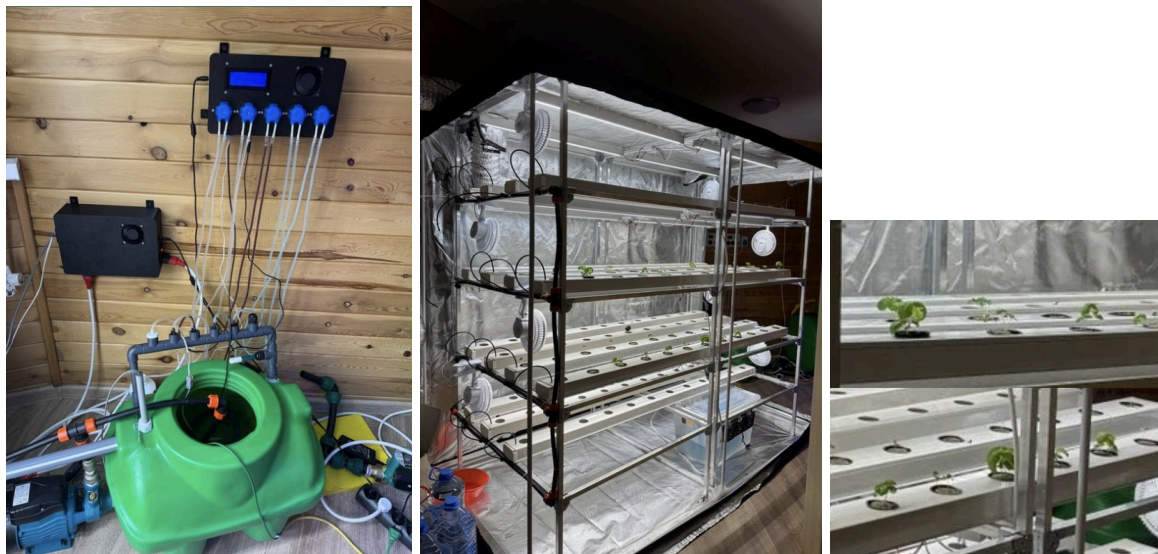
Figure 14. Control systems and Growing bed with plants
