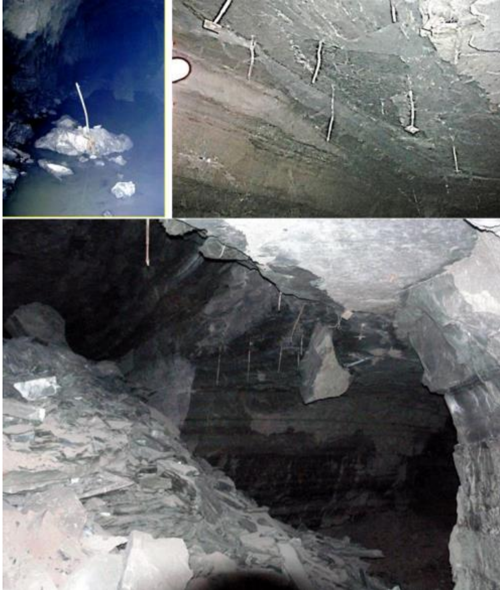
Figure 8. Types of roof failures in chambers at the Zhezkazgan deposit
