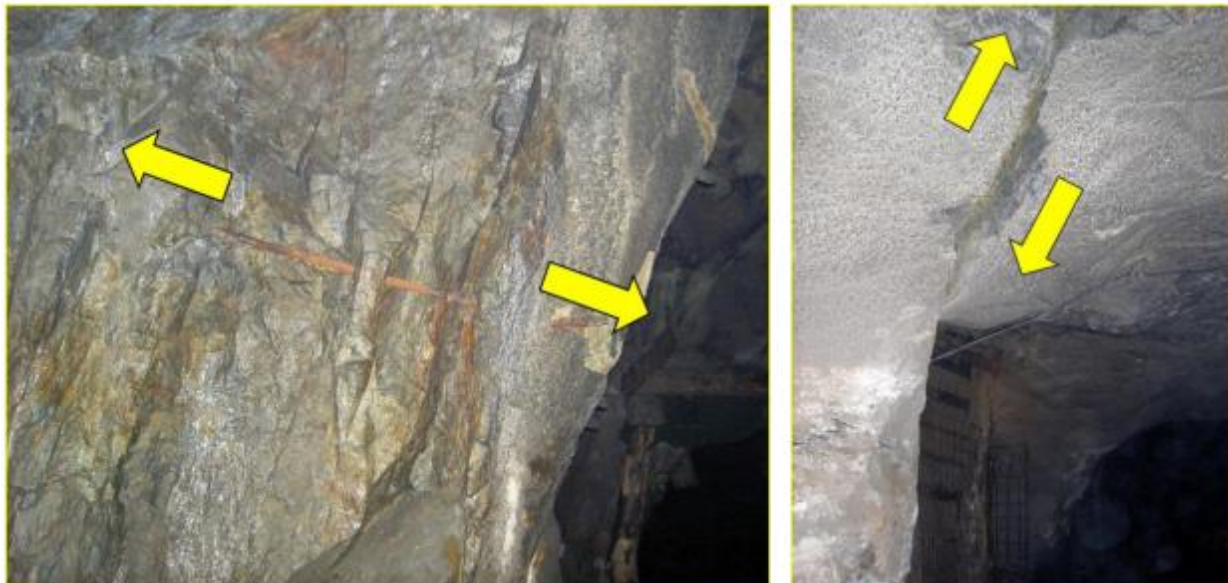
Figure 5. Formation of cracks on the lateral surfaces of pillars and in the roofs of chambers at Zhezkazgan deposit
