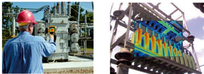
Figure 2.1: Thermography technology applied on transformer
