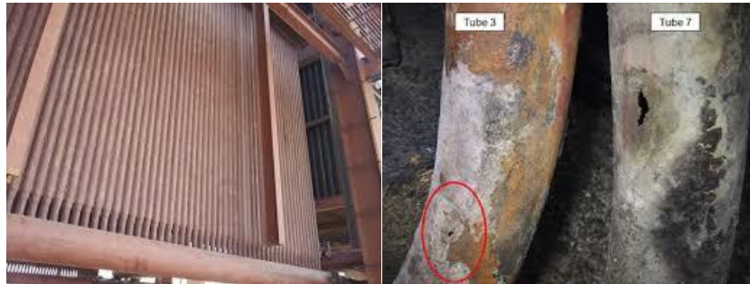
Figure 2.1: Boiler Tube Water Wall and Particular Tube Failures
